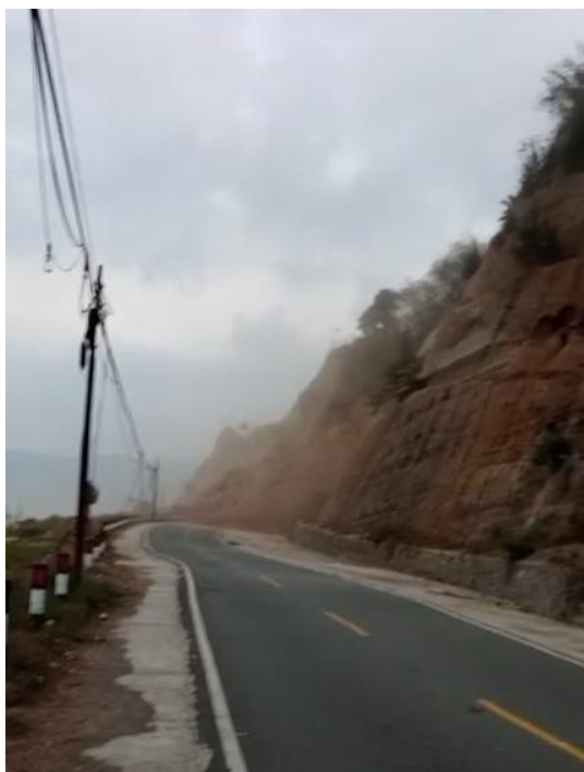
Figure 3. Landslide on the Trans Ende-Bajawa Road
