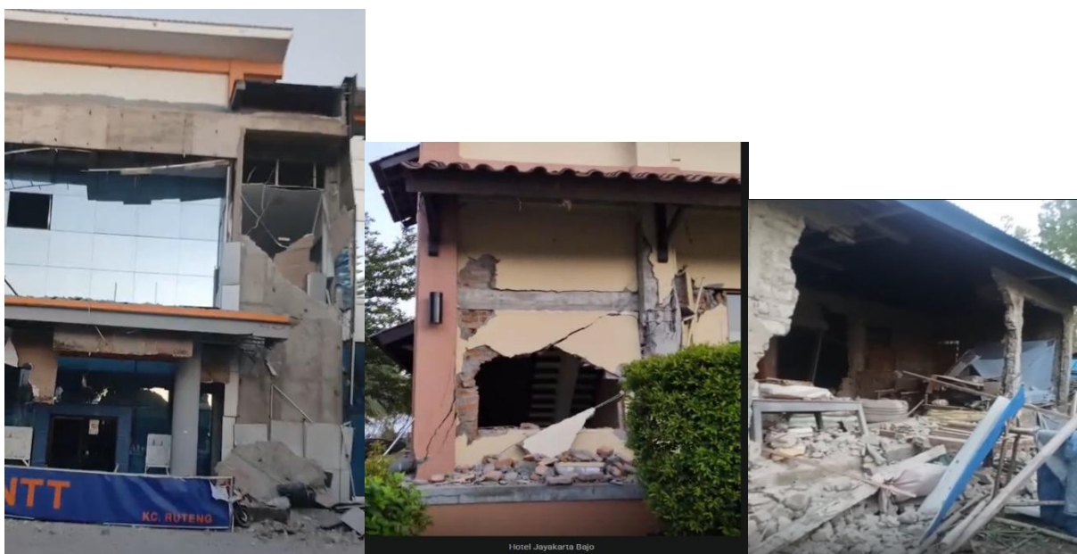
Figure 4. Damaged buildings in Manggarai and West Manggarai, NTT
