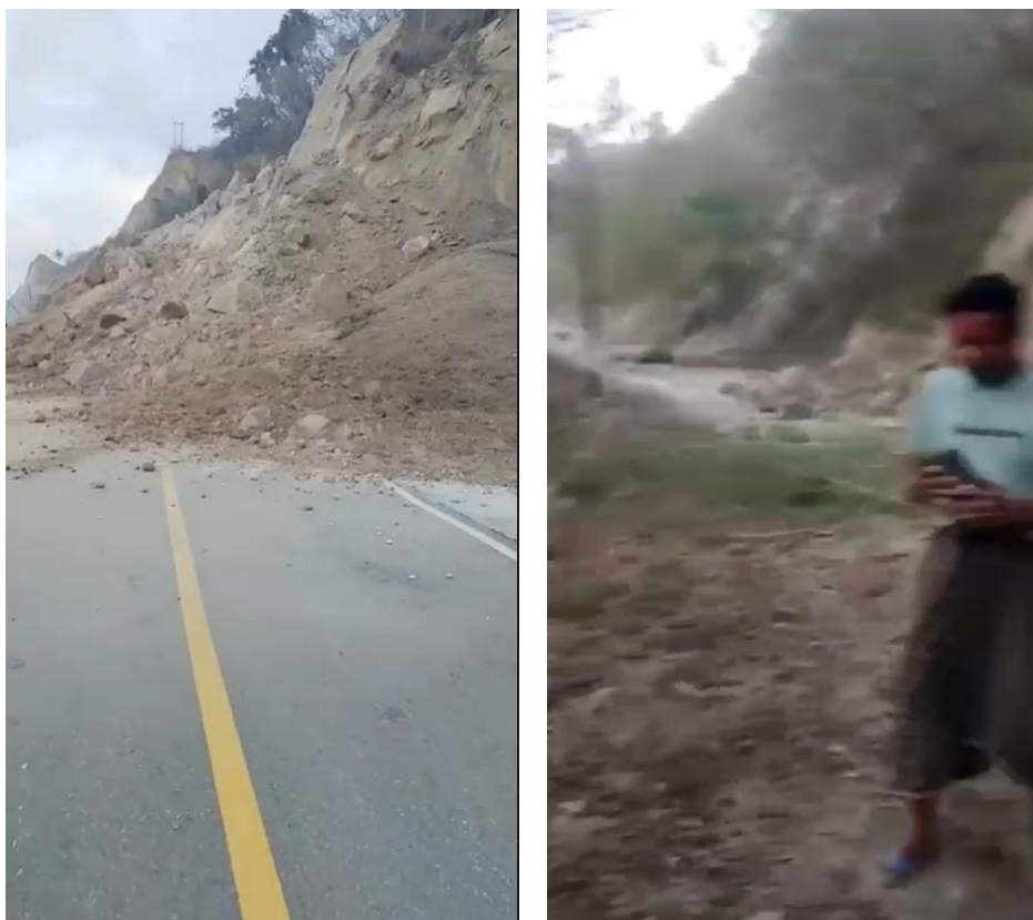
Figure 2. Roadblock from landslide caused from the earthquake in Ruteng, Manggarai, NTT
