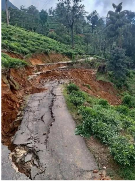
Fig.3.1: Road Damaged by Landslide, Paragala, Sri Lanka
